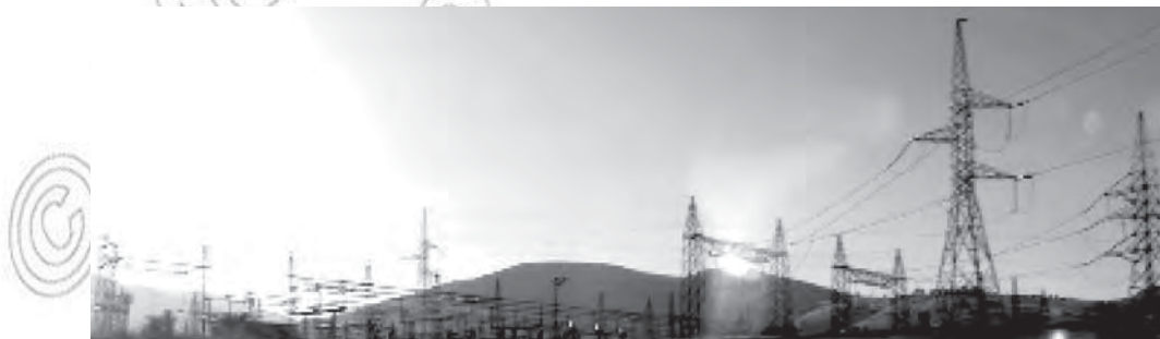
High voltage power lines and pylons
